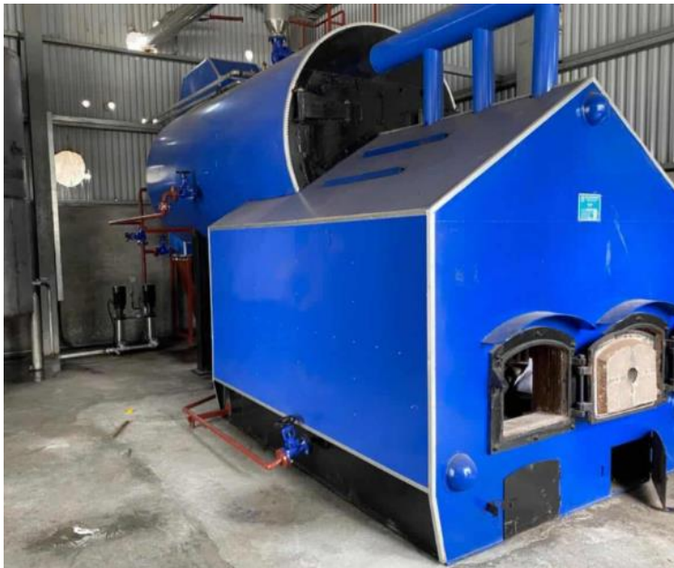
Boiler fix chain grate
